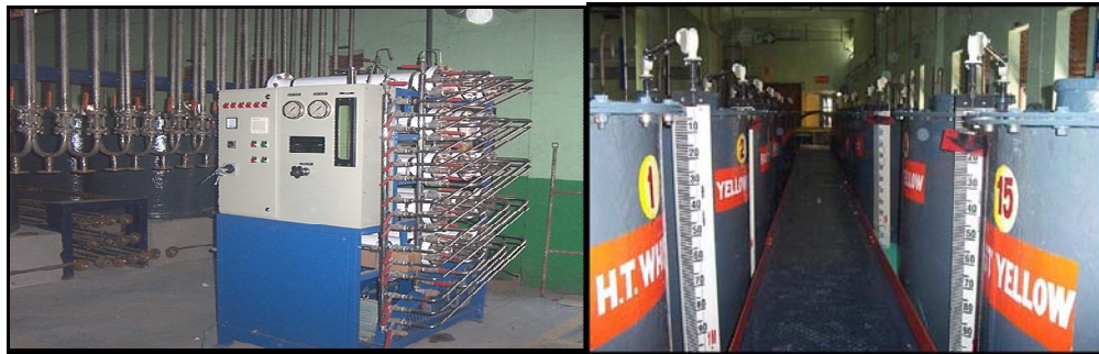
Ultra filtration of AMC washes water and Storage tanks
