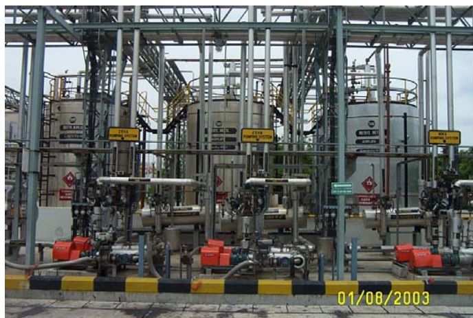
Bulk Storage Facilities - Monomer Tank Yard
