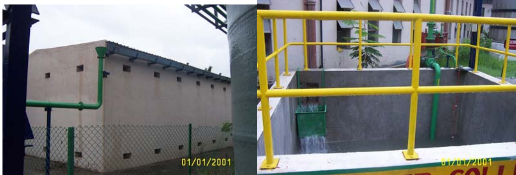
Rain Water Harvesting System-1.Roof Top Collection 2.Intermediate Storage
