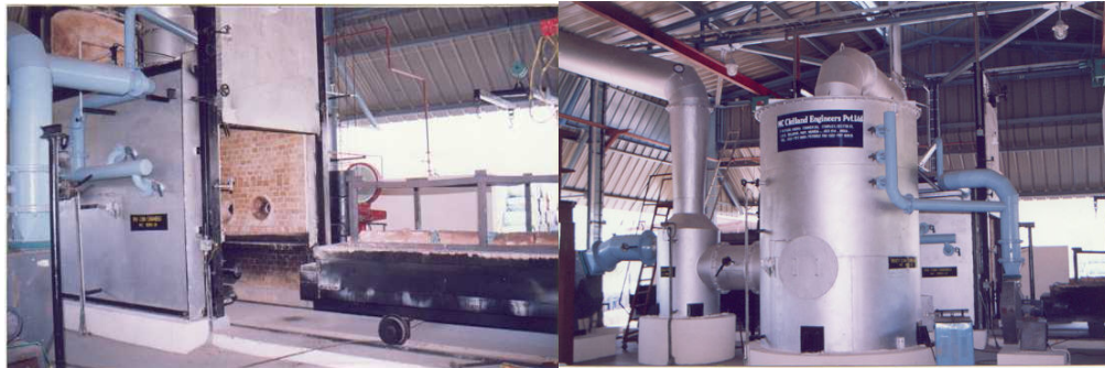
Primary and Secondary Chambers of Incinerator
