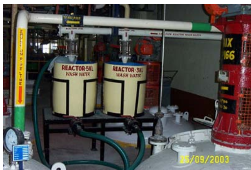
Emulsion Wash Water Reuse System
